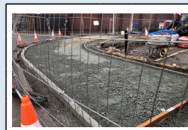
26/1/18 - Footway being constructed to meet the new multi-storey car park vehicular entrance
