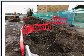
7/3/18 - The water pipe has been extended & relocated from the retaining wall location
