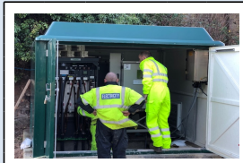
5/1/18 - The electricity substation being energised.
