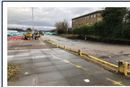
20/2/18 - Day 2 on site, excavation starts to the shrubbery bank for the retaining wall.
