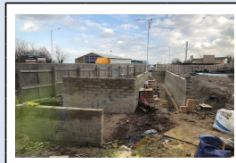
7/3/18 - Facing brickwork being installed to the ramp and staircase off of Eurolink Way
