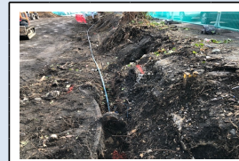
6/3/18 - Another unknown metal structure encountered that the water pipe is running through
